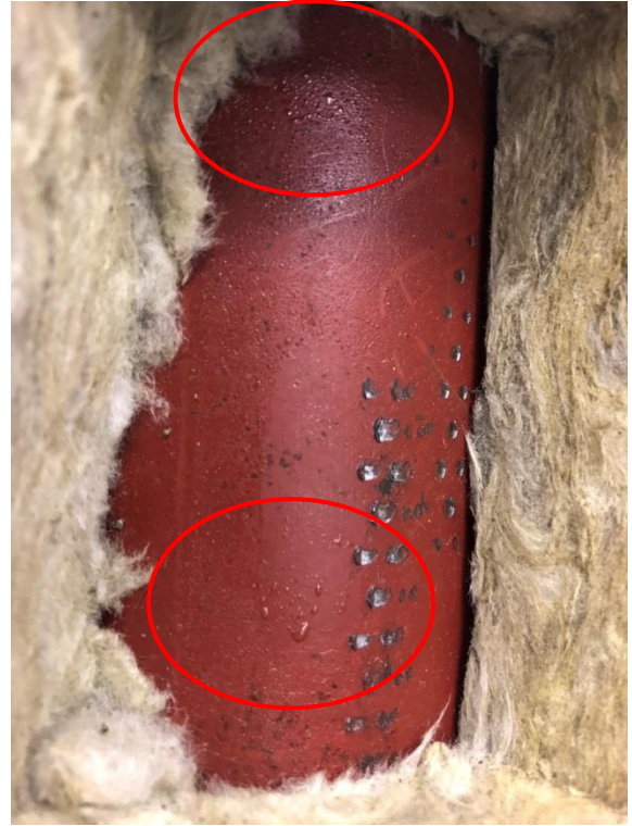
Figure 5 Condensation on the pipe covered with System 2 at the end of the two hours exposure
