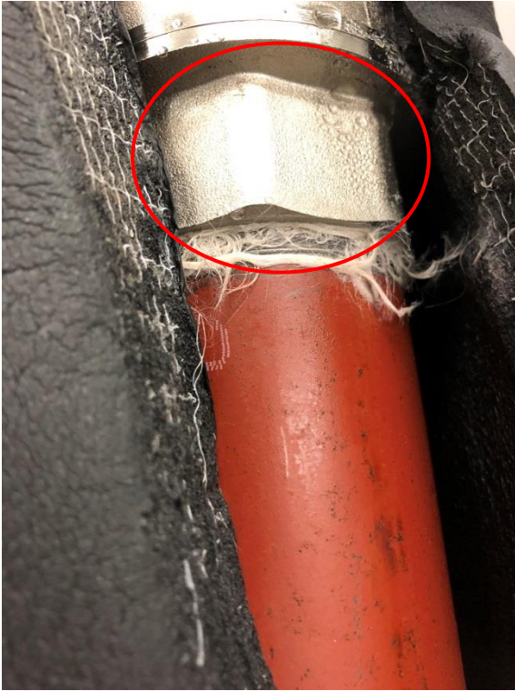
Figure 4 Condensation on the pipe covered with System 1 at the end of the two hours exposure
